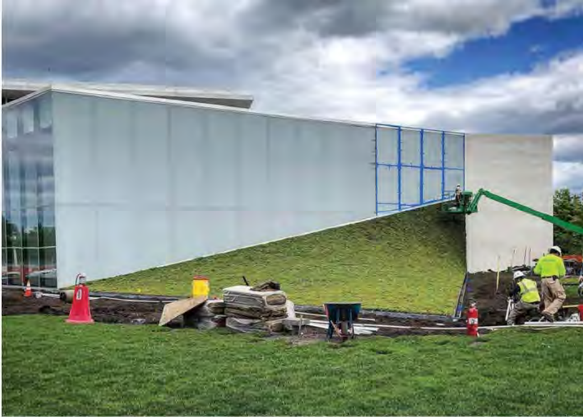
Hydrotech's GardNet and other components of its sloped garden roof assemblies were used in The Reach - the John F. Kennedy Center for the Performing Arts' recent expansion project in Washington, D.C. In several areas, the roof slope's geometry twisted from flat to vertical like a corkscrew. Photo courtesy of Hydrotech
